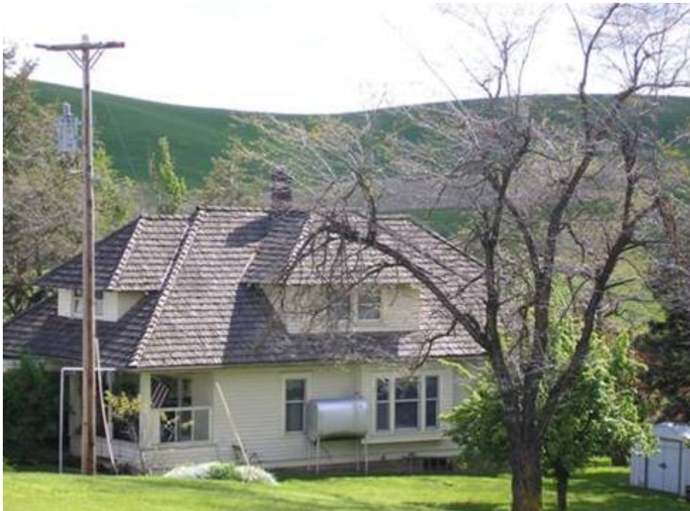
Heating oil tank (AST)
