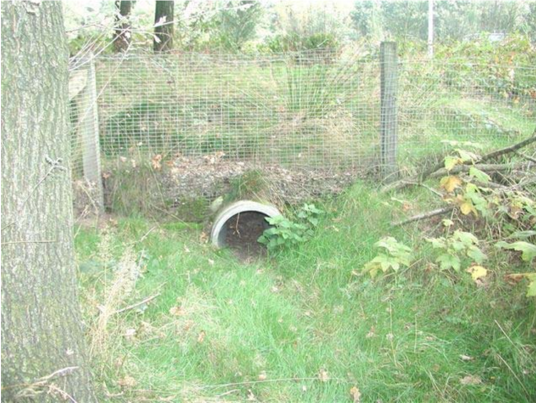
Figure 2. Badger tunnel with small animal fencing (Netherlands). Suitable for small mammals, reptiles or amphibians. Author recommends 36” or 48” box culverts for common mid-sized species.
