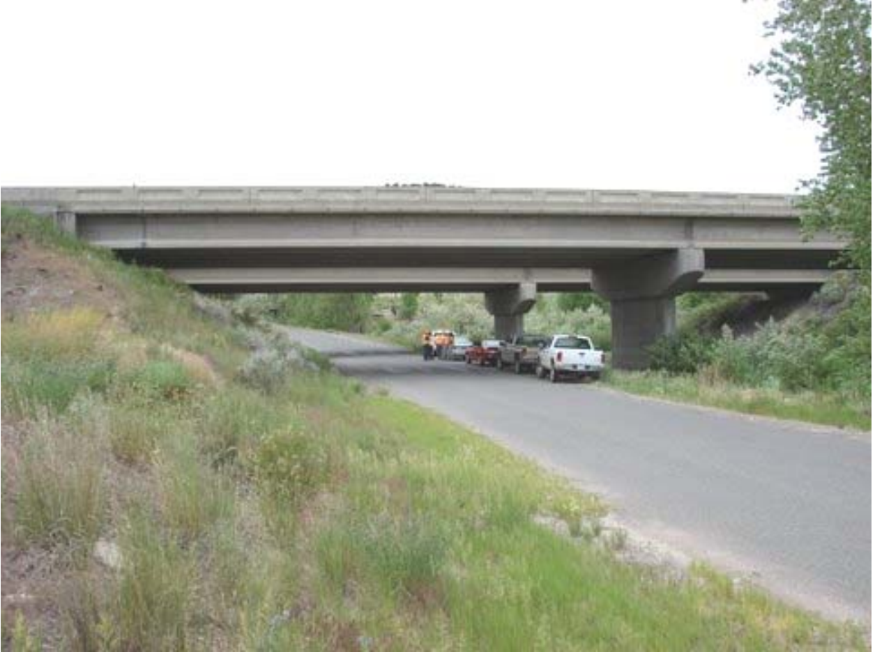
Figure 3. Country road crossing (twin spans) of US 6 near Price, Utah. This structure serves as an effective vehicle and wildlife crossing. Note the natural soil/vegetation on the sides of the bridge and the adequate length of the structure.
